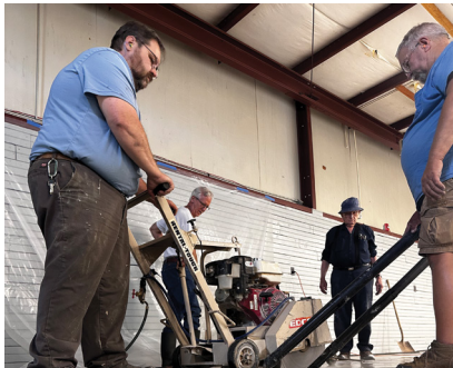
Jonathan Cutting Concrete While Marvin Looks on in Preparation for a Reinforced Pad for the Press — Photo by Dan Winder
